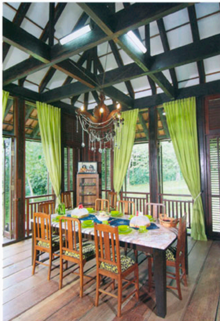
Up above, the exposed chengal structural beams serve both form and function in a network of very good joinery work, providing a visual feast of lattice-like pattern from certain angles.
